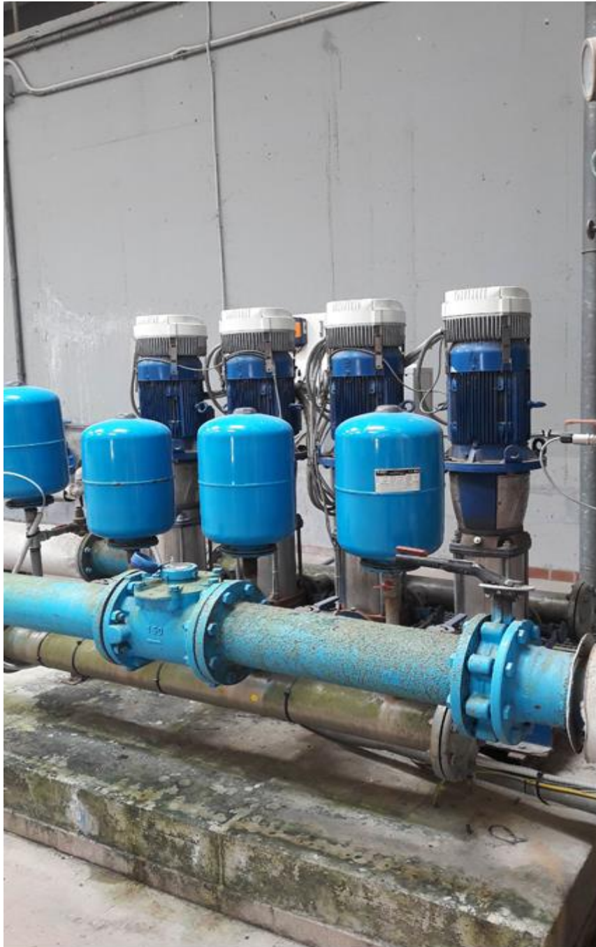
Cargo City Drinking Water Station
