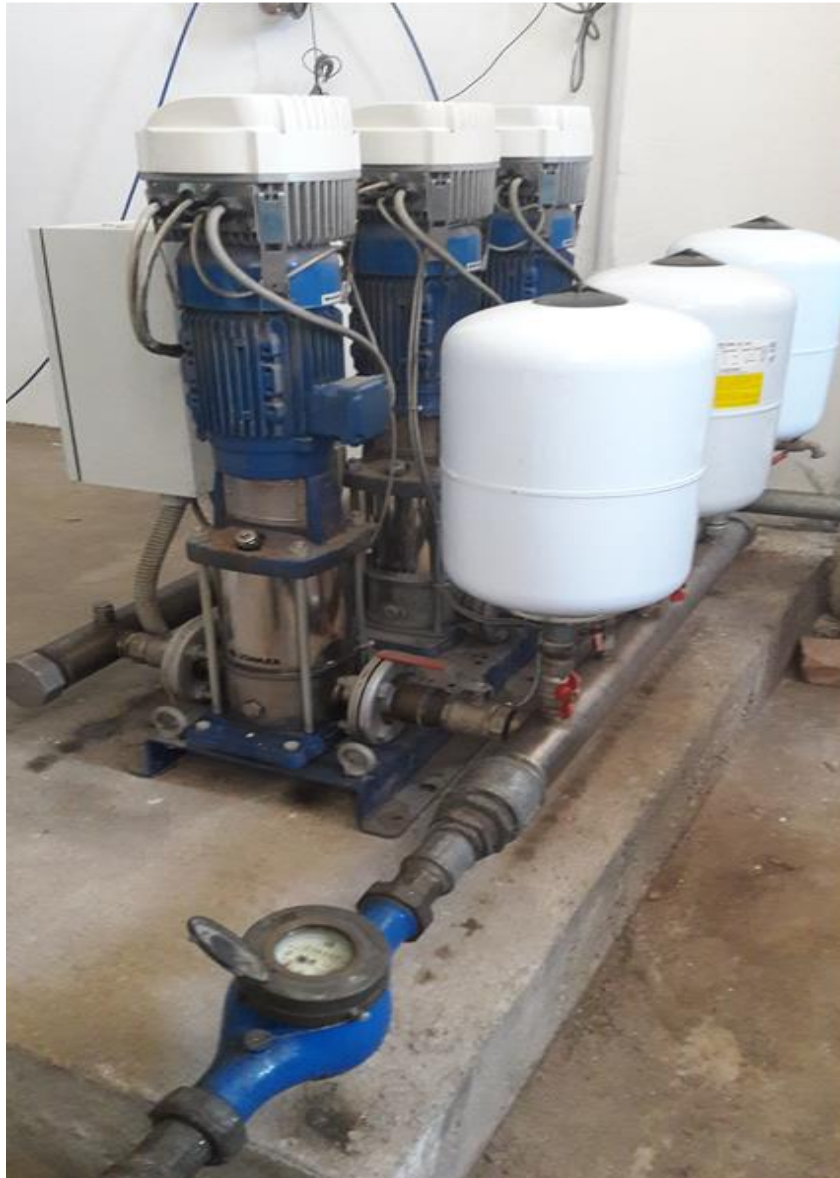
Central Cafeteria Drinking Water Station
